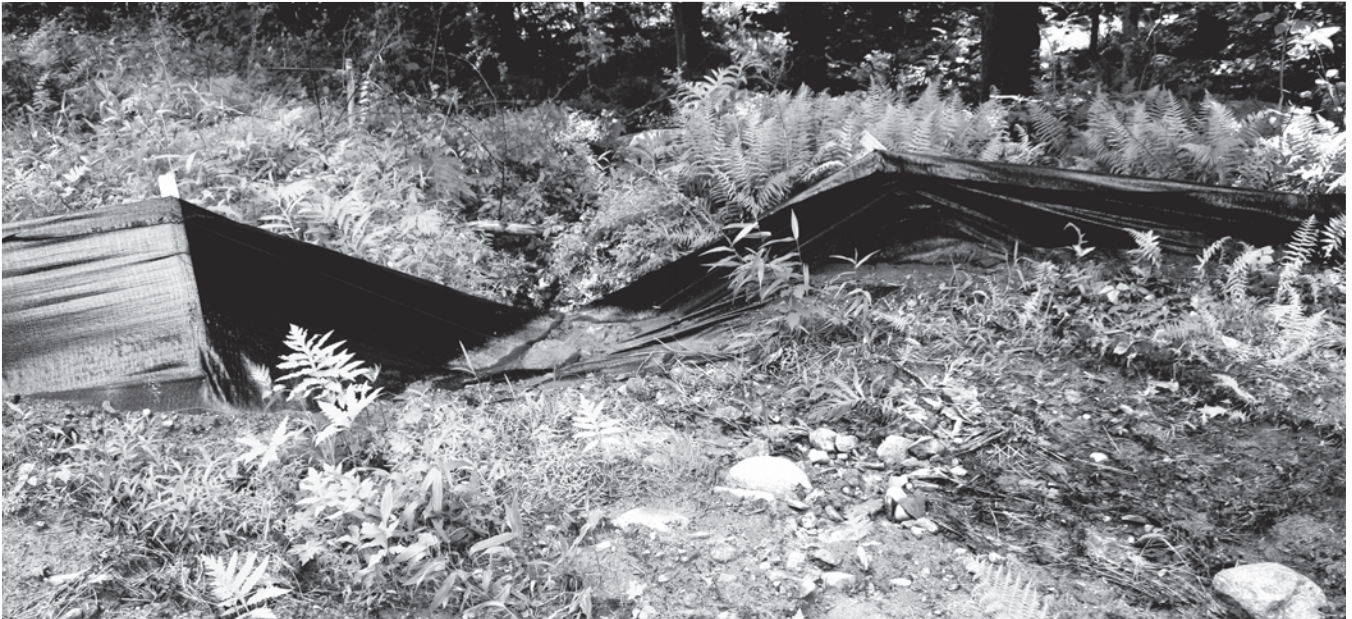
Filter fabric silt fence overtopped by storm runoff, Algonquin Pipeline, Town of Yorktown, Westchester County, New York, 9 July 2014. Erik Kiviat © 2015.
